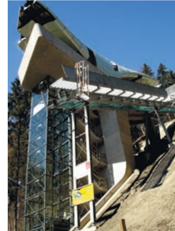
Hungerburg Funicular, Innsbruck, Austria, Zaha Hadid, 2006. Alpenzoo Station during construction with most of the glass panels installed. Photo courtesy of design to production
