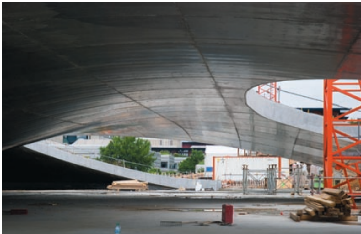
The small shell after taking out the formwork. Photo courtesy of designtoproduction
