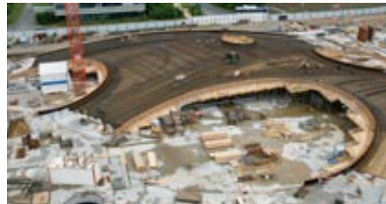
Formwork during assembly. On the left part the rebar are already in. Photo courtesy of designtoproduction
